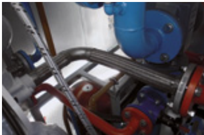
Stainless steel hose in a combined heat and power plant with 90° bend with swivel flanges on one side and welding ends at the other side.
